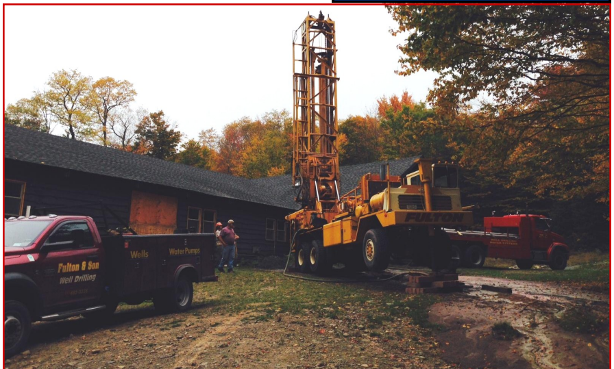
Drilling of the Council House's new well both commenced and finished on Sept. 30.
