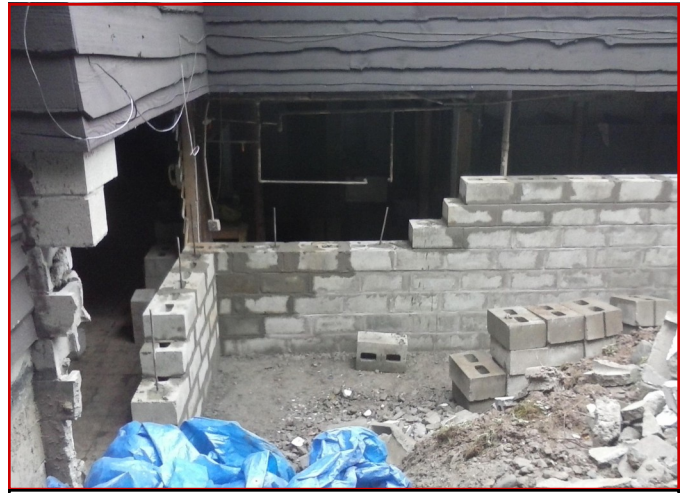
The north side of the Administration Building experienced significant renovations in the month before the OAA's 2014 Fall Weekend.
